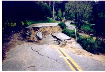
Road damage due to landslides in 1997-98 El Nino winter in Santa Cruz Mountains –
